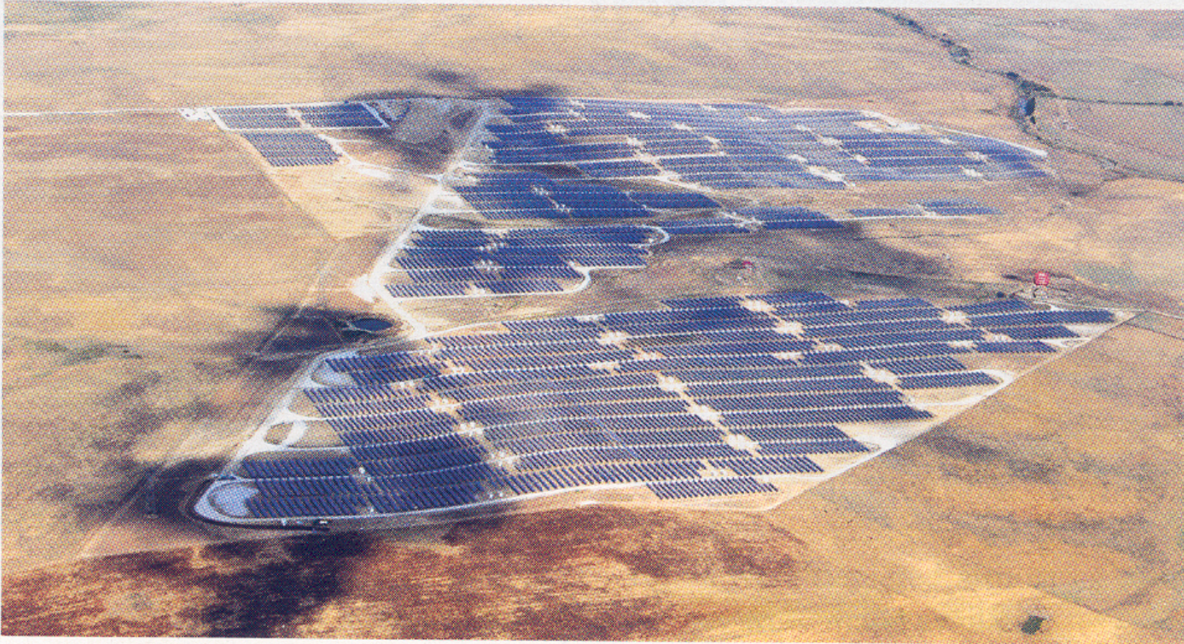
A 23.3 MW solar park in Trujillo, Extremadura, Spain. Photo courtesy of Suntech.
