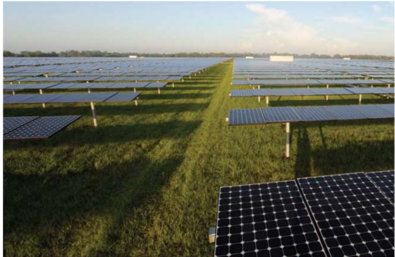
Florida Power & Light DeSoto Project (25 MW PV) in Central Florida - Commissioning Fall 2009
